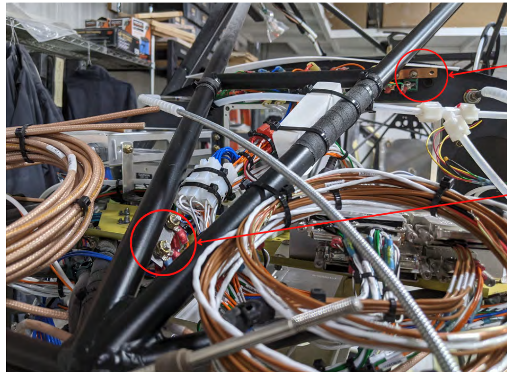
Figure 18 - Panel Wiring Front View
