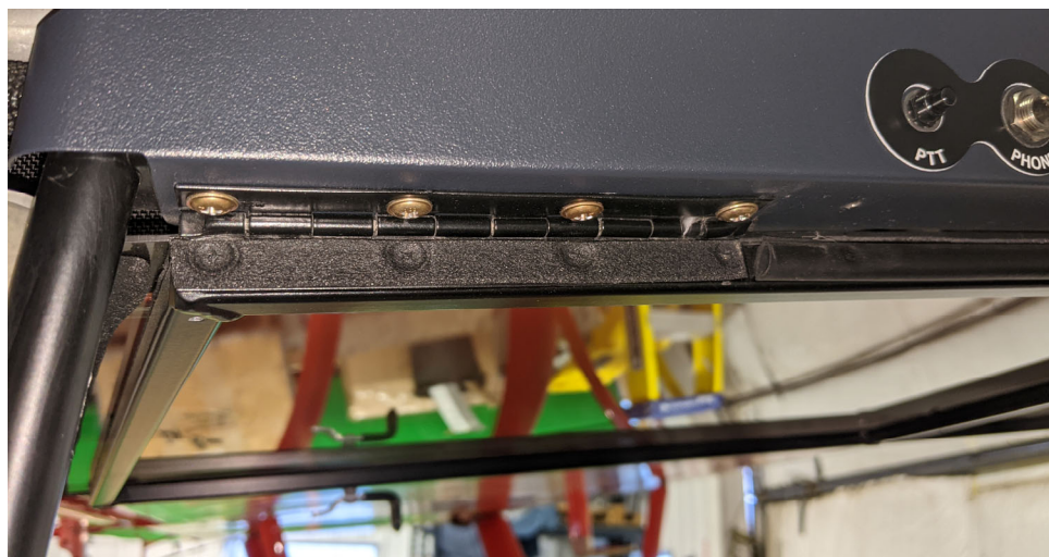
FIGURE 5 – Foam Seal on Window Hinges
