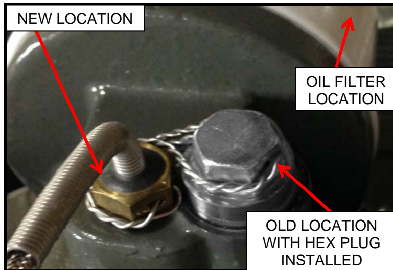
FIGURE 6 - Probe and Hex Plug Installed
