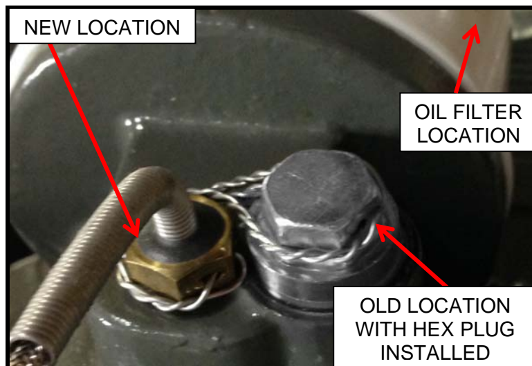
FIGURE 5 - Probe and Hex Plug Installed
